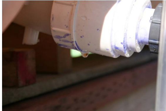
Small leaks caused by joint stress due to flexion of secondary tanks.
