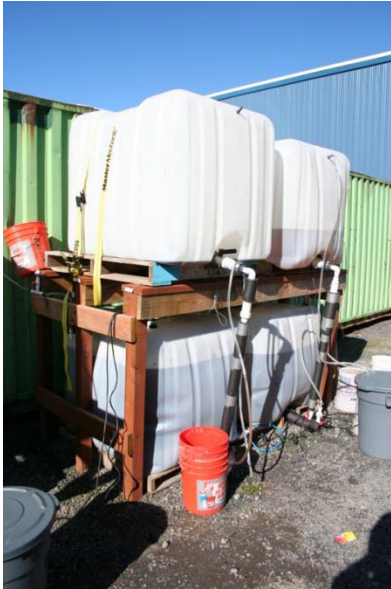
Current configuration of secondary water-pressure tanks with attached pump buckets. Weathering on the tanks has caused considerable lead and distention.
