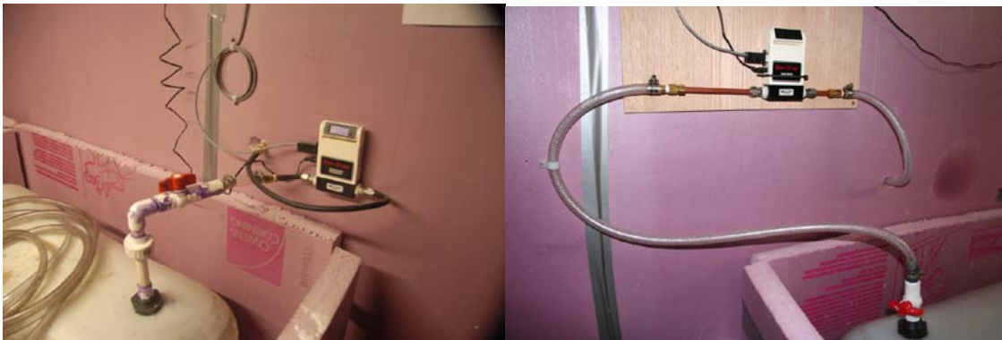
Figure 8. Pictures representing the old and newly installed gas outlet systems. The old system (left), which was originally installed on February 19, 2011, was demonstrated to have several leaks common among multiple tanks. The decision to retrofit and install the new system (right) was made on January 9, 2011, following a teleconference among project team members at the CEC boardroom and UAF. The new install was completed as of February 25, 2011.
