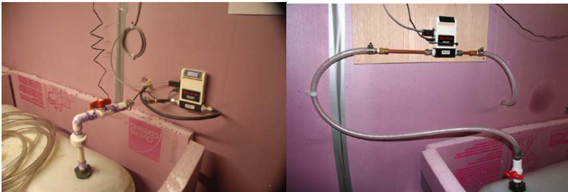
Figure 8. Pictures representing the old and newly installed gas outlet systems. The old system (left), which was originally installed on February 19, 2011, was demonstrated to have several leaks common among multiple tanks. The decision to retrofit and install the new system (right) was made on January 9, 2011, following a teleconference among project team members at the CEC boardroom and UAF. The new install was completed as of February 25, 2011.
