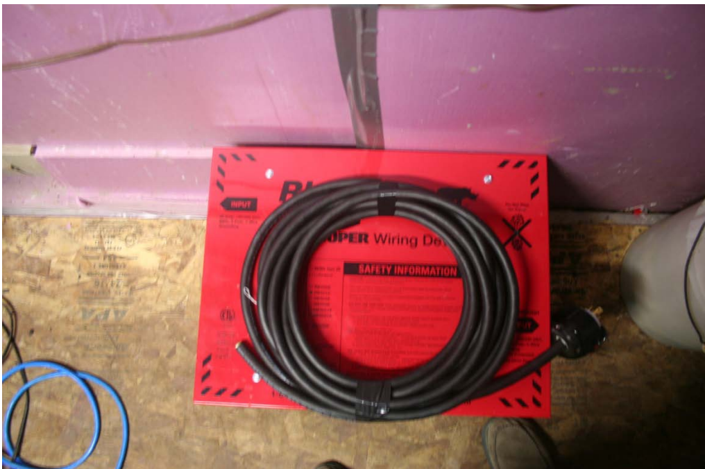
Once installed, this Rhino™ Spider circuit will be used to power the Connex. This system will be a significant improvement on what is currently in place and will conform to any state or local utility regulations as well as improve the overall electric consumption of the project.
