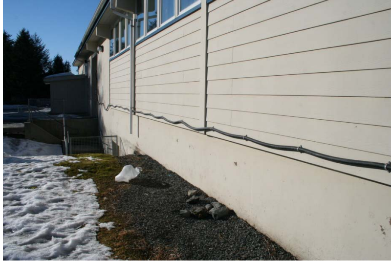
New power cable installed to route additional power to the project site. March 8, 2011.
