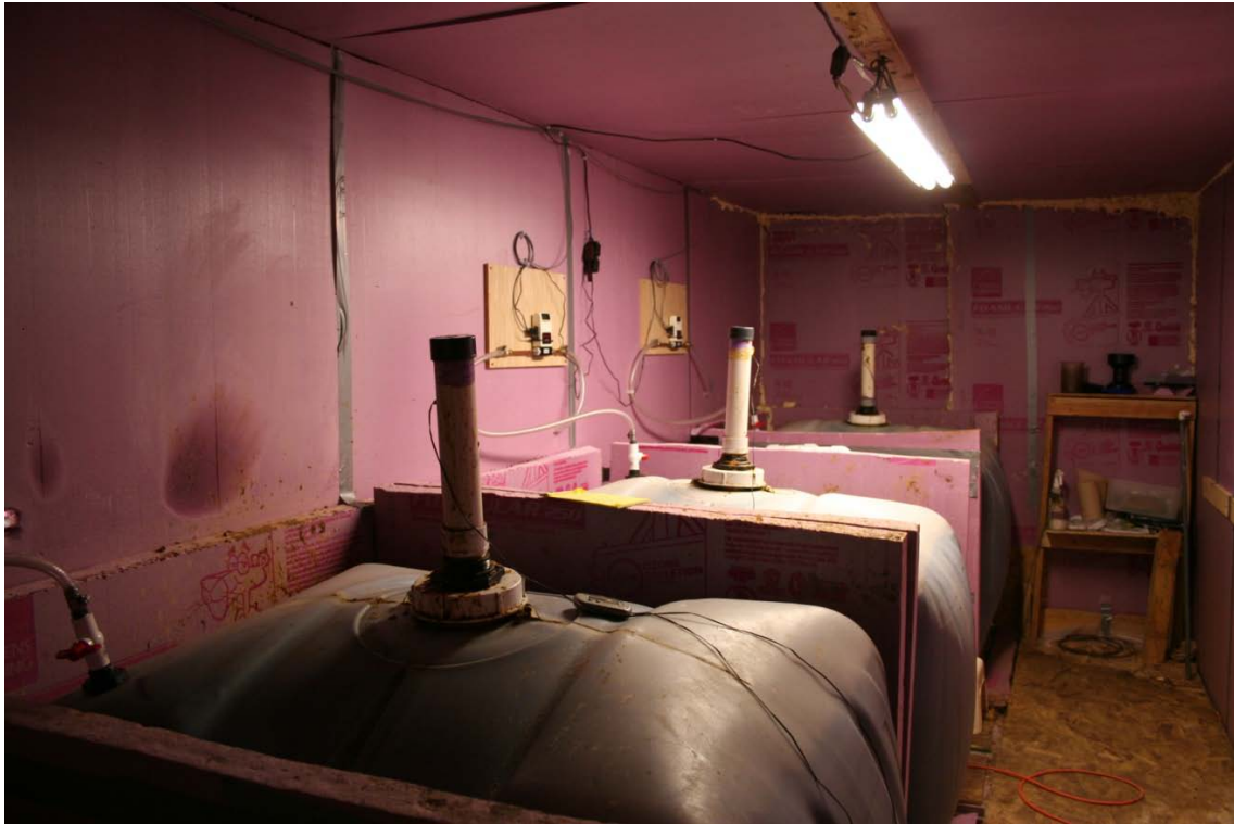
Flowing the install of new gas outlets among all of the tanks in the 25°C room each tank began demonstrating the ability to hold pressure. Here each tank is pictured accumulating biogas prior to a venting.
