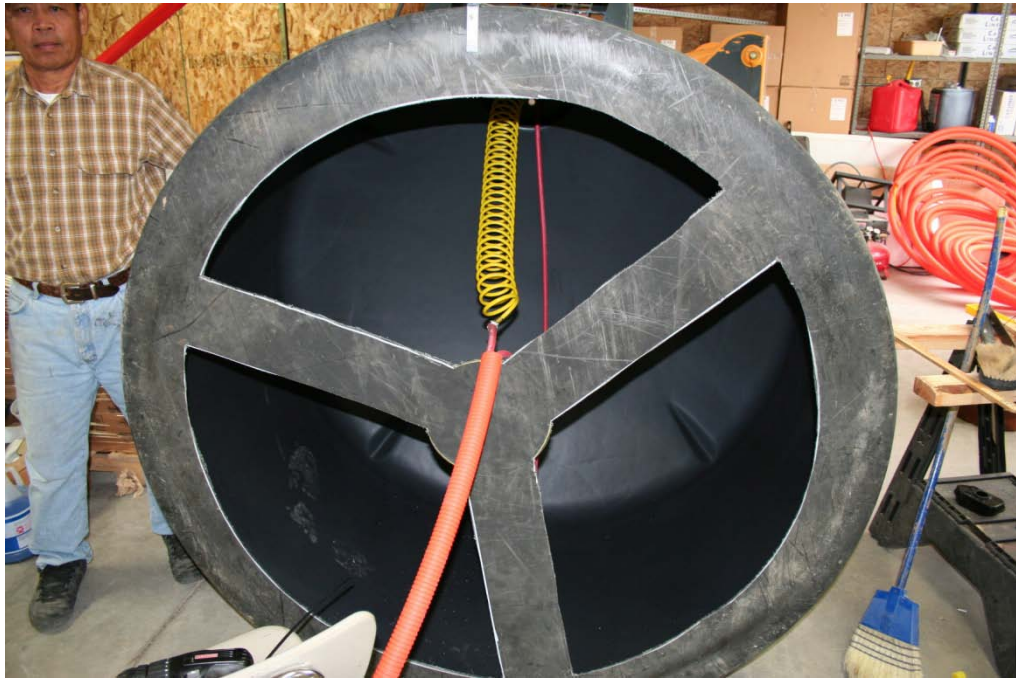
The completed storage tank, prior to being assembled inside of the larger containment vessel. CHS Janitor Romey assists in the assembly within the Cordova Energy Center, located at CHS.
