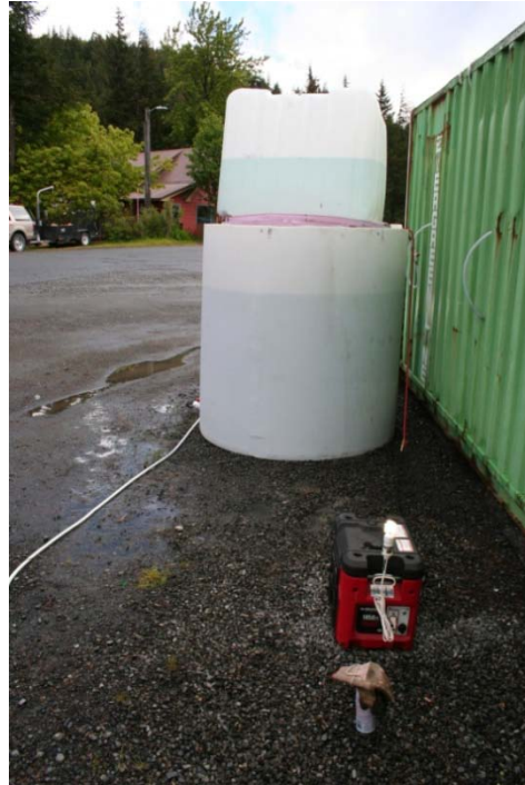
Biogas being used to power a generator. Note the additional water weight used to increase the pressure of the gas supply for running an electrical generator. The water weight was not required for cook stove operation on biogas.
