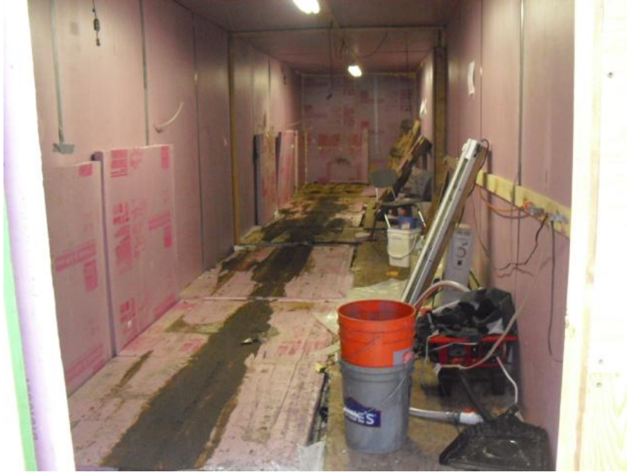
Final project site as of July 18, 2011. Insulation and lighting arrays remain to be removed at the school districts discretion. Photo credit: Clay Koplin.
