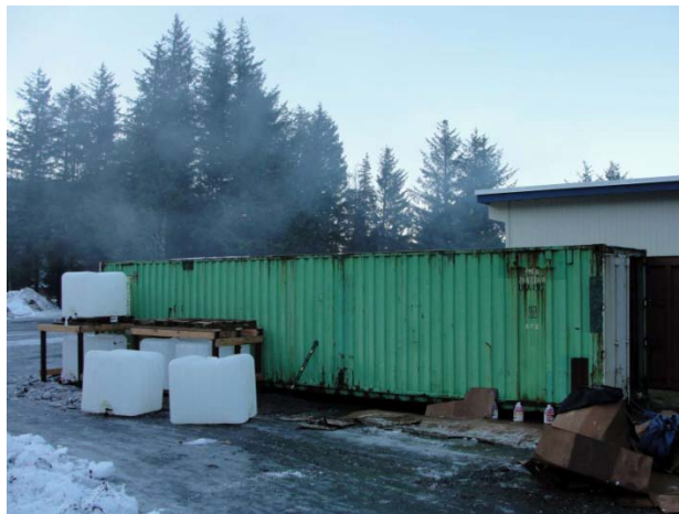
The Connex in first stages of construction behind CDHS, with water pressure tanks outside.
