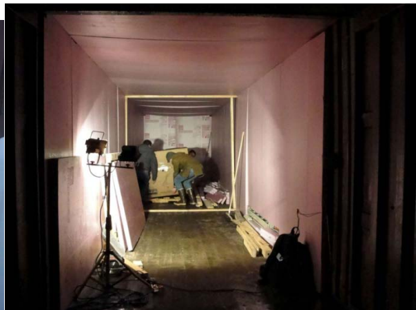
Insulation panels going up inside the Connex, while McFadden and Culhane place the primary slurry tanks.
