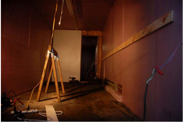
The dividing wall between cold and warm rooms goes up, while electrical wiring is installed.
