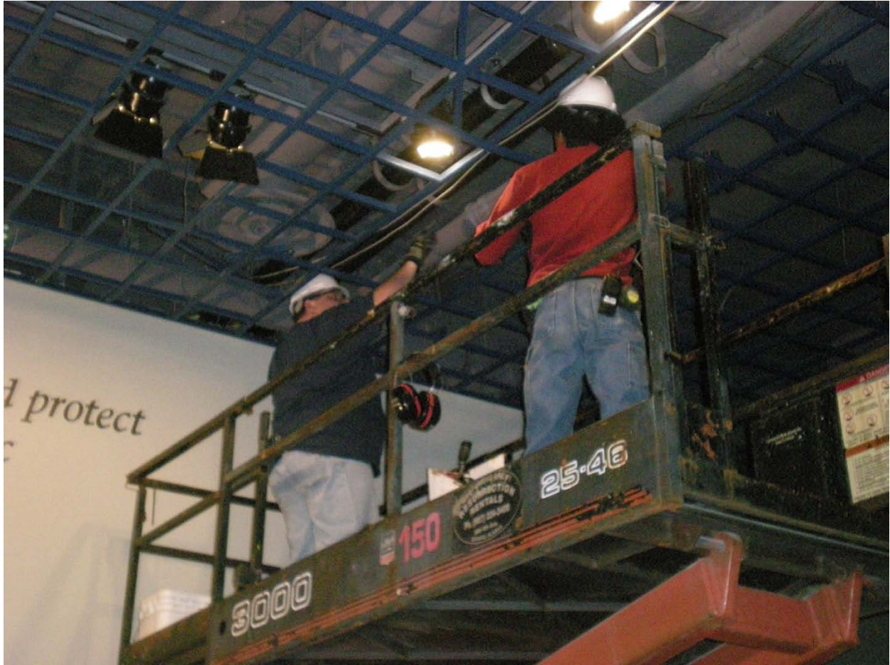
Figure 8 ASLC LSS Group Manager John Underwood and LSS Technician Isaac London installing Victaulic heating loop piping - April 5, 2011
