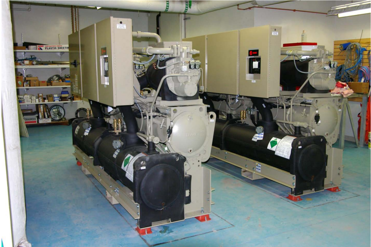
Figure 5 Trane heat pumps installed in ASLC boiler plant room - March 18, 2011
