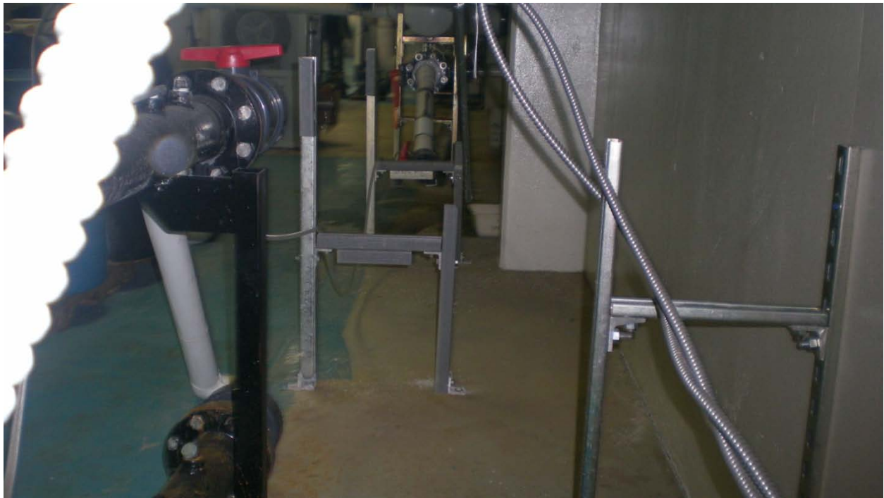
Figure 4 Pipe Corridor for Condenser and Evaporator Loop Piping
