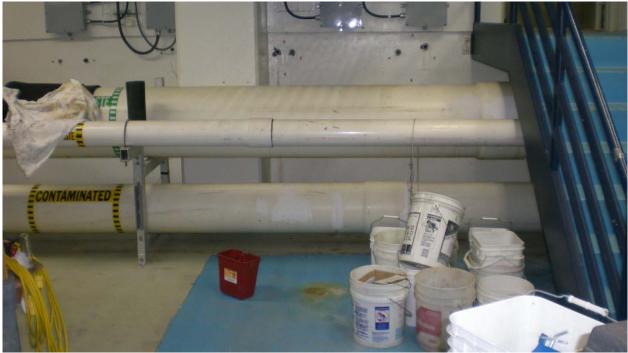
Figure 7 Location for Titanium Plate Heat Exchanger - HX 3
