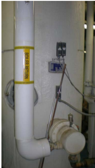
Figure 9 Domestic Hot Water Tank
