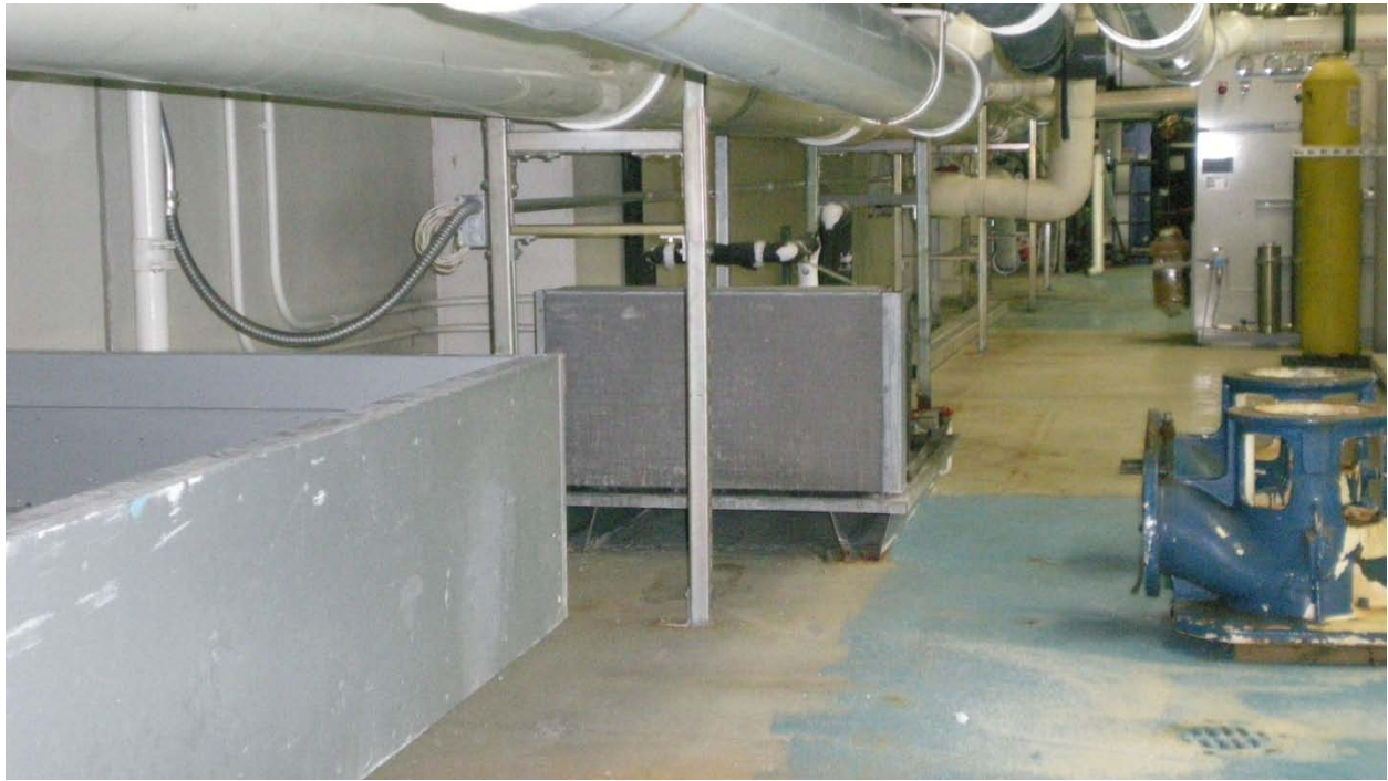
Figure 5 Corridor for Condenser and Evaporator Loop Piping
