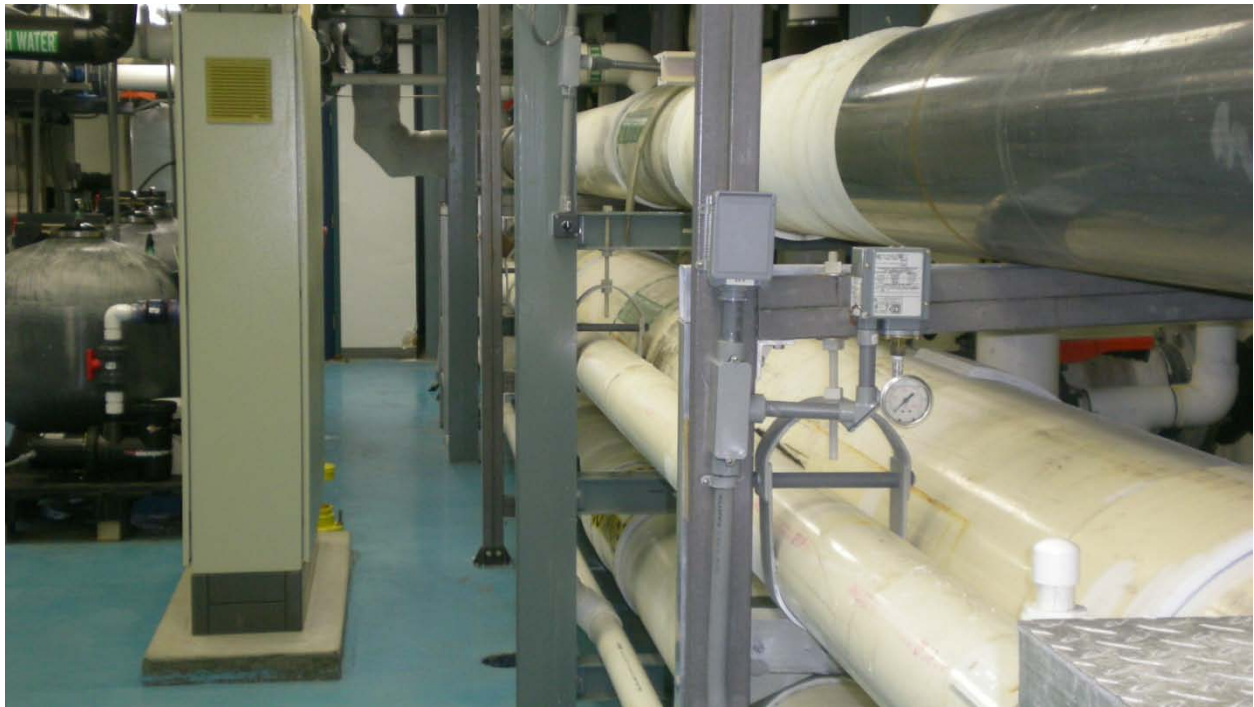
Figure 6 Corridor for Condenser and Evaporator Loop Piping
