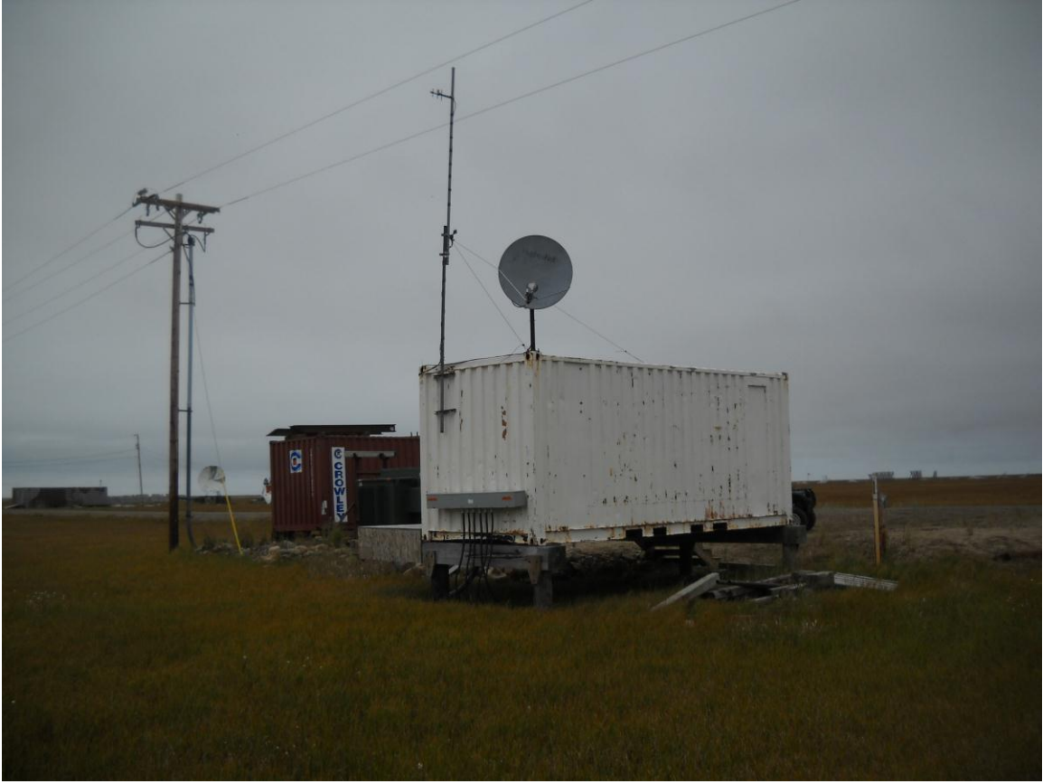
Picture 2: Control connex with newly mounted HughesNet satellite internet dish.
